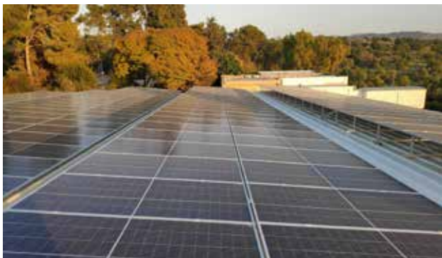
Solar panels – Aran Israel
